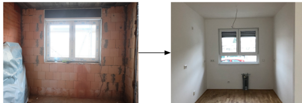
Figure 1: The two photographs show a construction site at an early and late stage in the construction progress.
